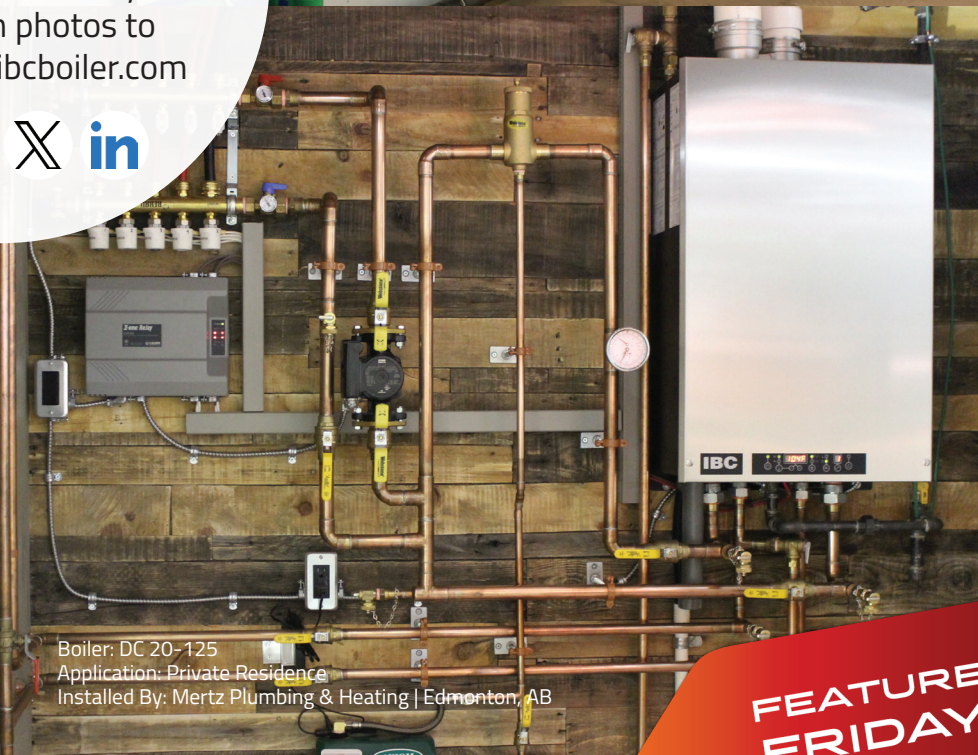
Products: SL 80-399 x 5 Application: Hydronic Heat to Forced Air Radiators Installed By: Gleeson Plumbing, Inc. | Moorefield, ON
